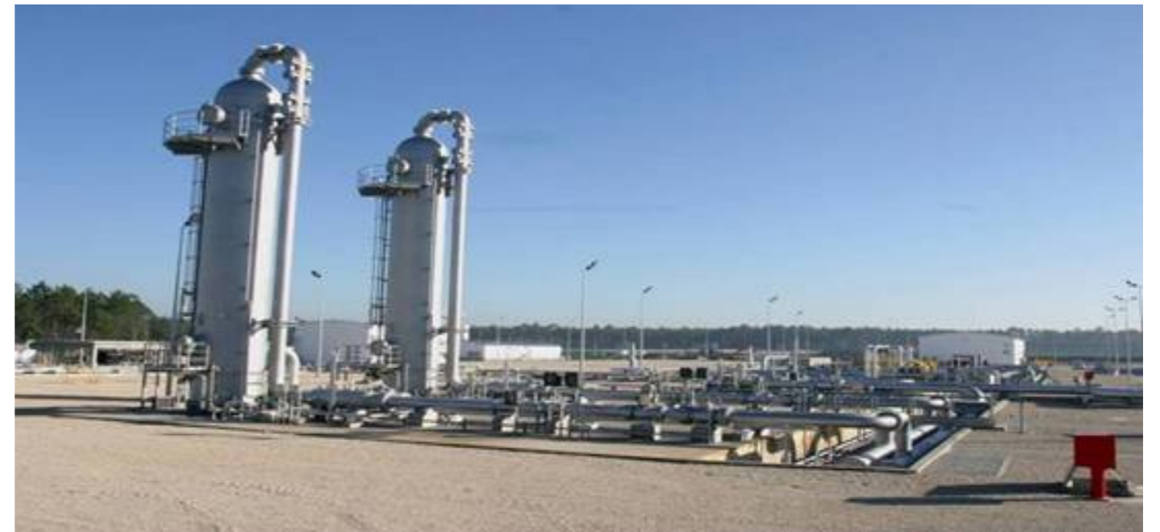
Figure 28 - Installation de surface du stockage souterrain de gaz naturel de Carriço. ( https://www.ign.ren.pt/arrazenamento-subterraneo3 )
